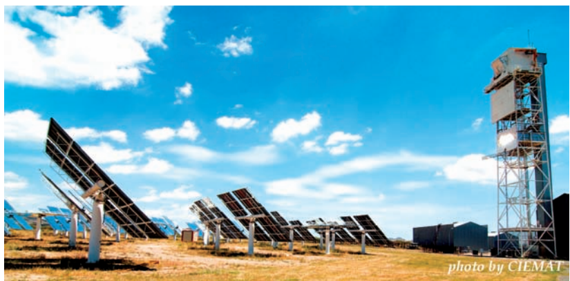
Figure 20.9 The thermochemical solar hydrogen plant, with the solar tower where the scaled up HYDROSOL II reactor is installed at the Plataforma Solar de Almería, in Spain.
